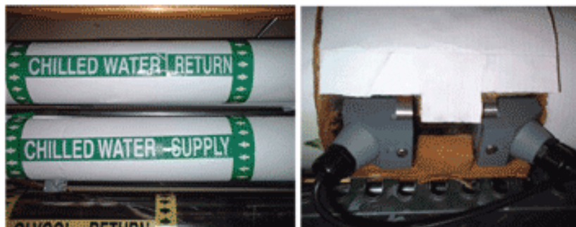
A set of clamp-on ultrasonic transducers mounted on a chilled liquid system.
