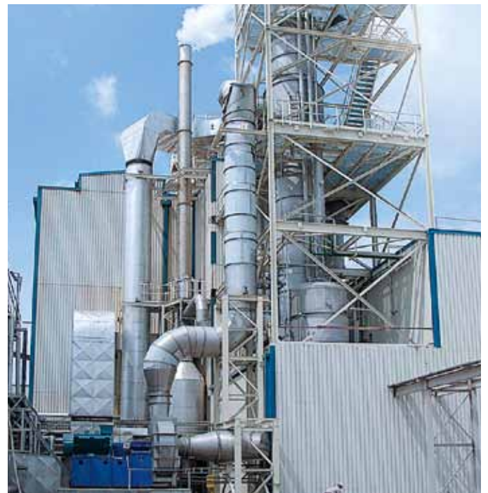
1-effect falling film evaporation plant heated by mechanical vapour recompression for wheat starch effluent. Evaporation rate: 17,000 kg/hr
