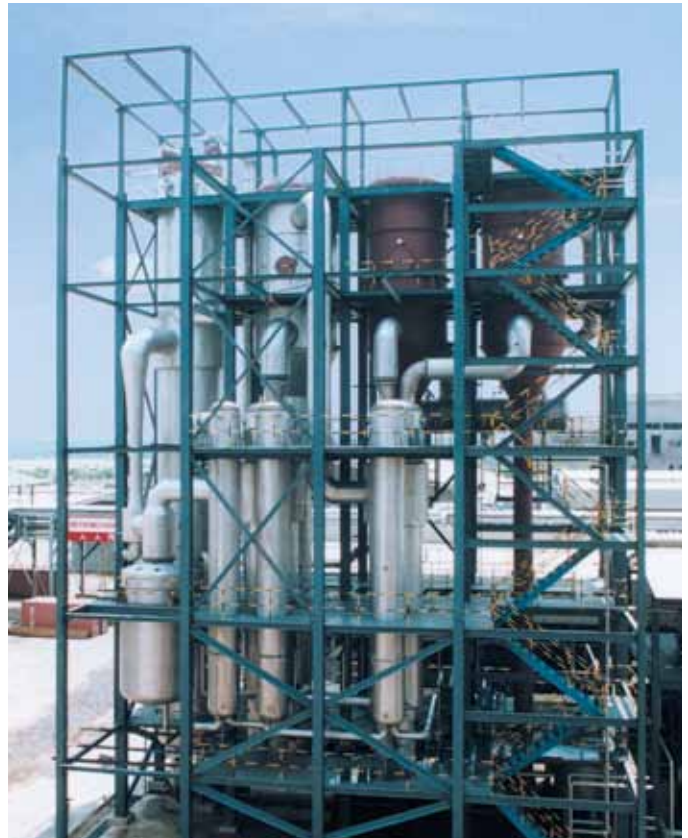
3-effect falling film forced circulation evaporation plant heated by thermal vapour recompressor for waste water from sodium glutamate production. Evaporation rate: 50 t/hr
